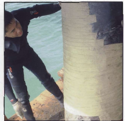
3. Strips of Densyl Tape are then placed over the Denso S105 Paste to bring the repair area up to the surrounding level.
