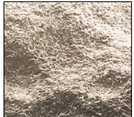
● After HoldTight Application: 15x magnification of dry blasted steel plate showing no contaminants.
